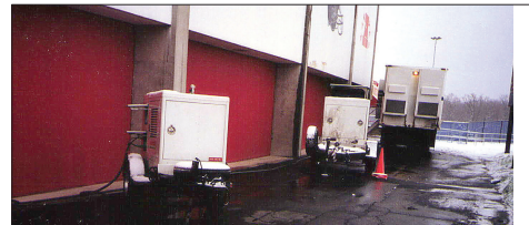
Figure 2.65 Parked truck with its backup generators nearby. (Source: Tim Stoffel)
